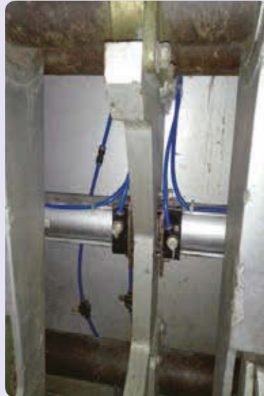
Automatic swing arms of sizing machines through technological improvement
